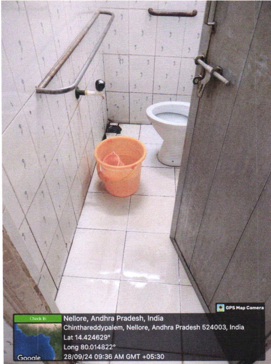
DISABLED REST ROOM
